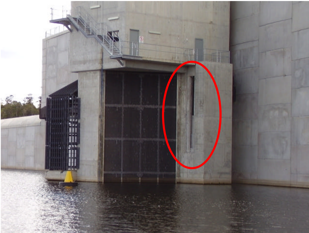
Image 3: Entrance to downstream fishway (vertical slot in red circle) 1 m above the water of the dam reservoir. Taken by Roger Currie on 11 May 2008.
